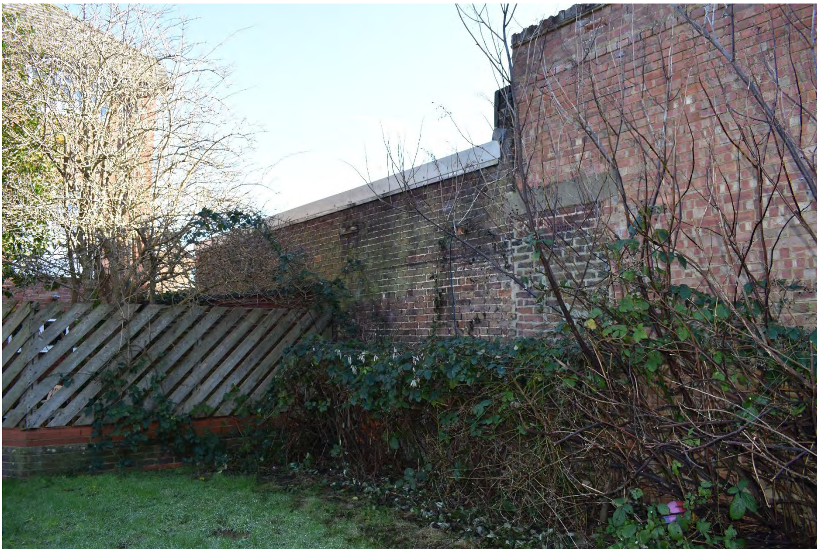
Plate 15: Rear view of the buildings on the northern boundary from Priory Grove (facing SE)
